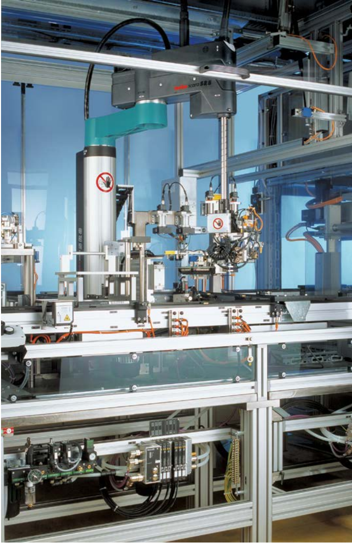
Flexible robot cell with transfer system
